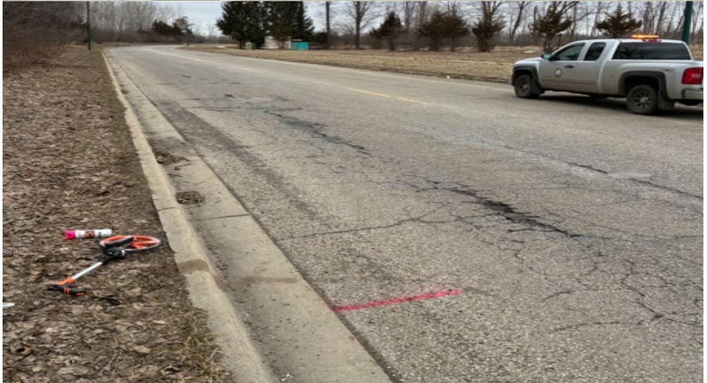
Reno Dr. between Robinson Dental and LS #7 West side of road Approximately 62 square yards
