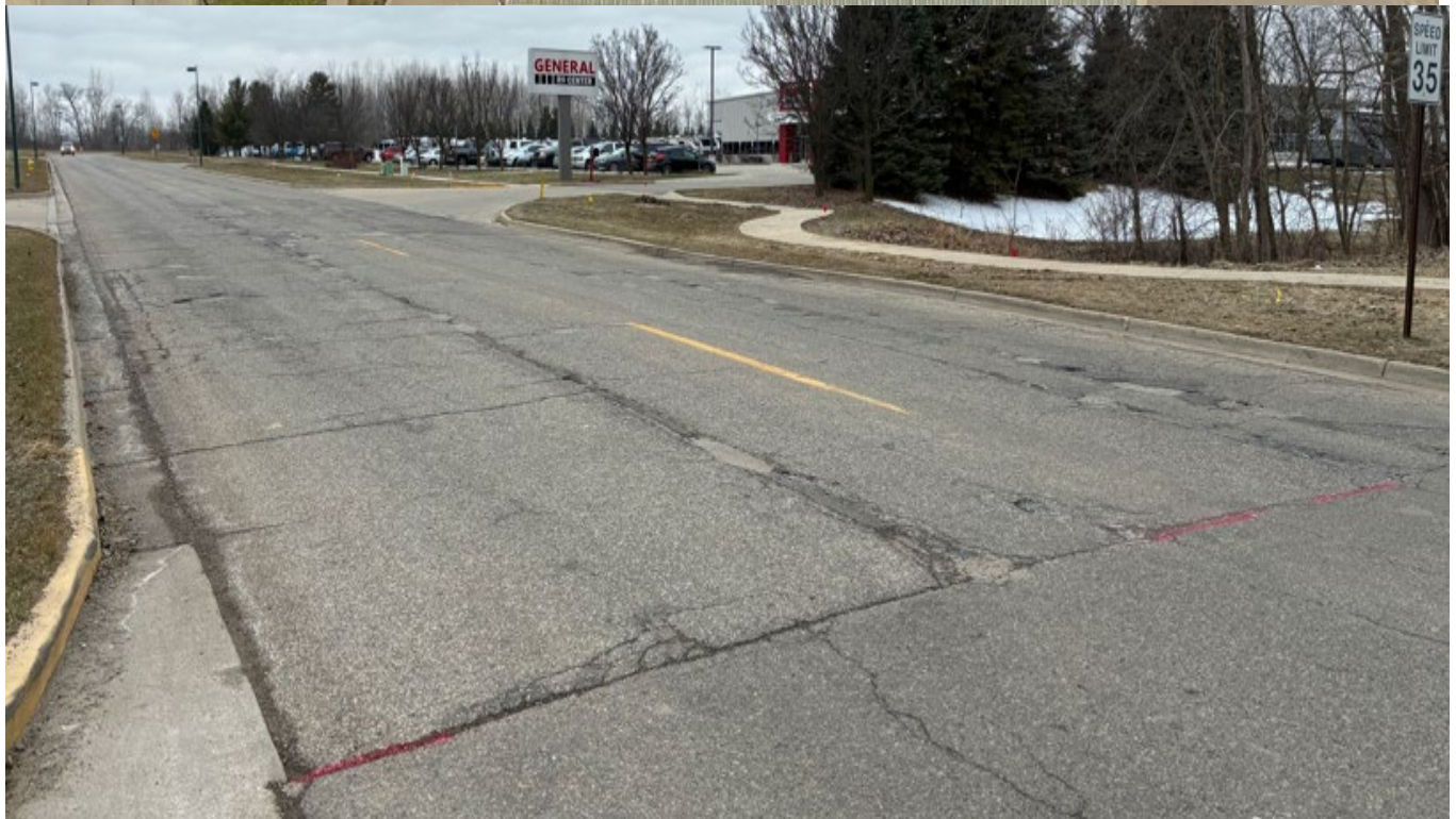
Reno Dr. from Do It Best to General Rv Both sides of road Approximately 575 square yards
