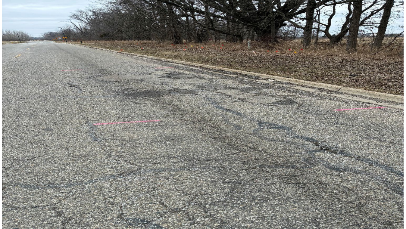
Reno Dr. North end of Robinson Dental, West Side of Road Approximately 32 square yards
