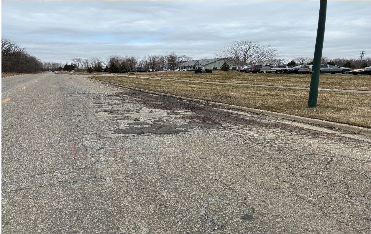
965 Reno Dr. East side of road Approximately 62 square yards
